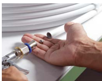
Ball Test To ensure that there are no occlusions or deformations on the inside of the pipe by using compressed air to pass a ball through the pipe.
